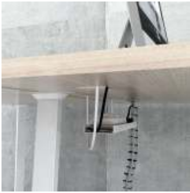
E64 HORIZONTAL CABLE TRAY
